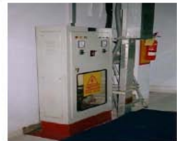
Electrical Panel Box
